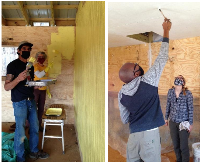
(Left) Varun & Lisa slather on a sunny yellow paint on the upstairs barn walls (Right) Lewis & Kat touch up a ceiling
