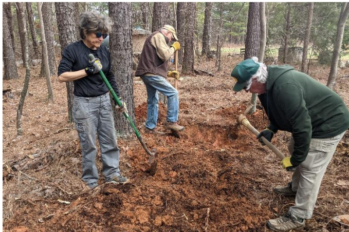
Kathleen, Paul, and Bill dig a trench at the workday (Photo: Shells)
