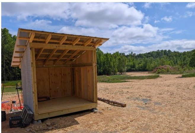
Anthony championed and coordinated getting two wellhouses framed and ready for the pump installation. (Photo: Hope)
